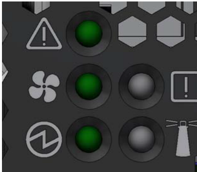
System Status LEDs* 5 Minutes After Power On
